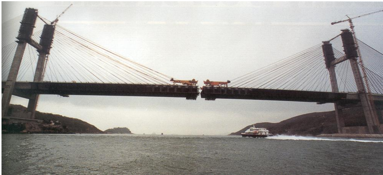
About to close the span, in March 1996, just ahead of Tsing Ma
