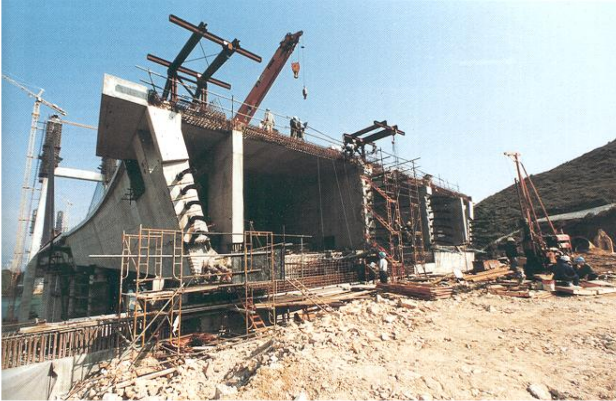
Lantau approach span launched into final position; probably the largest and stiffest incrementally launched
