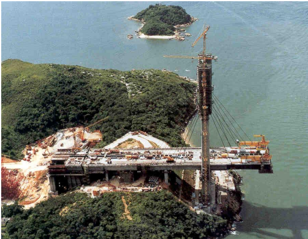
Ma Wan tower and approach spans, connecting to the Ma Wan viaduct (extreme left)
